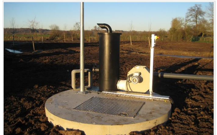
Outdoor NAT / Pumping station
