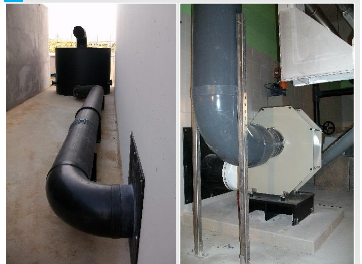
Outdoor NAT / WWTP
