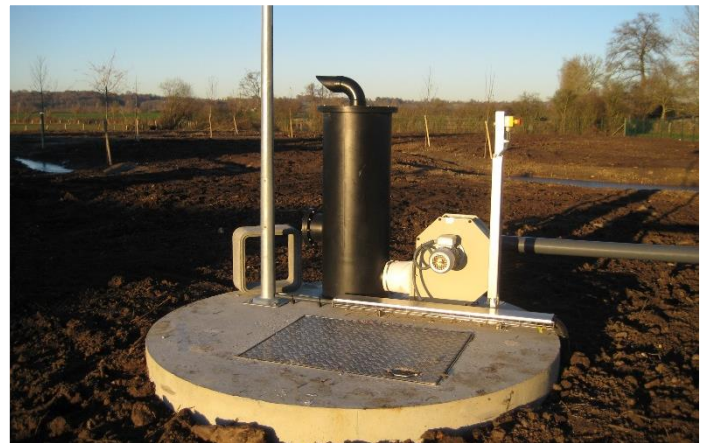
Outdoor NAT / Pumping station
