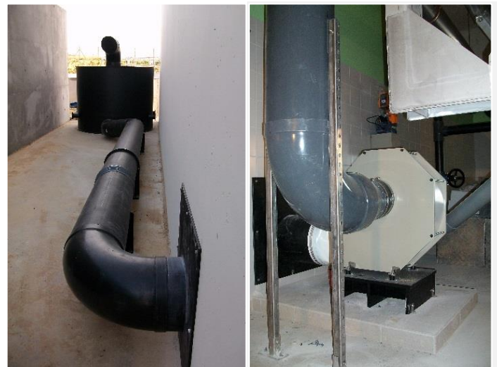
Outdoor NAT / WWTP
